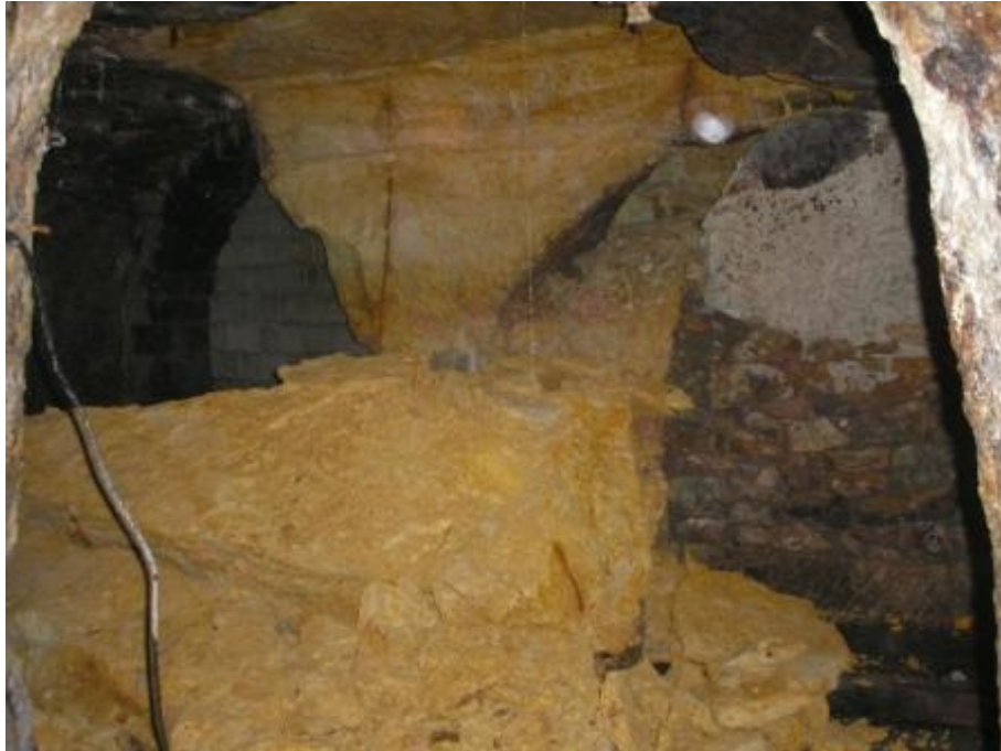
At least 30 m 3 rock collapsed here in Mád
