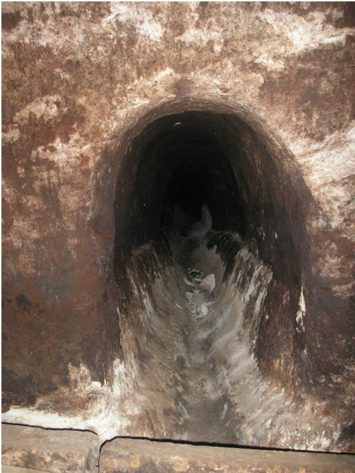
Drain for groundwater in Szegilong
