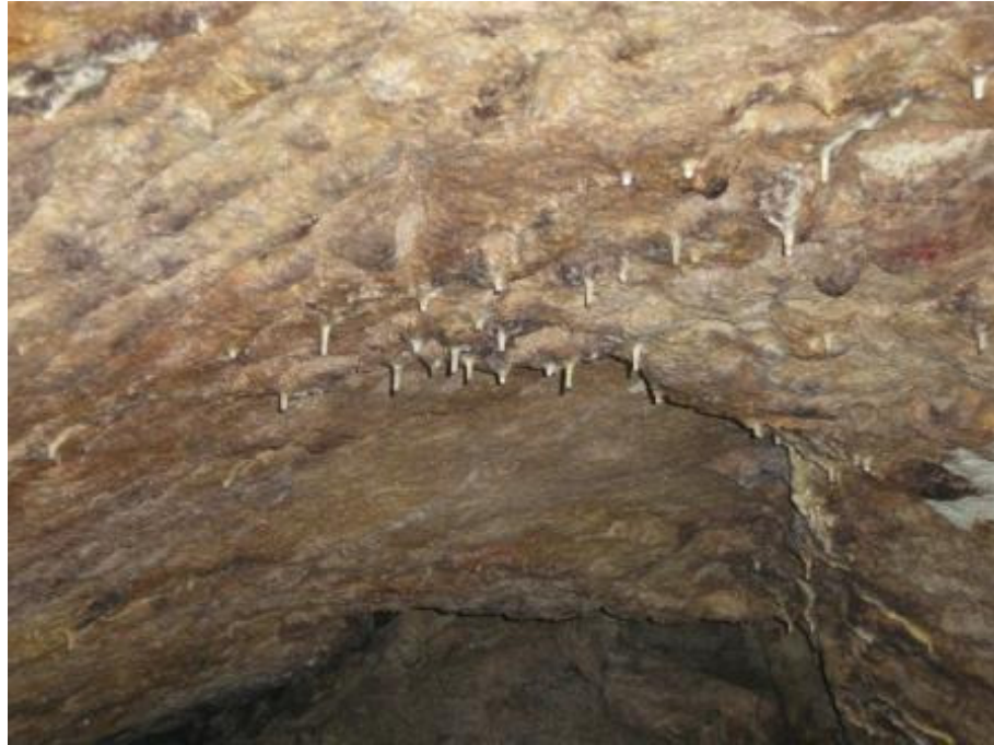
Stalactite formation in a cellar in Mád that is constantly leaking
