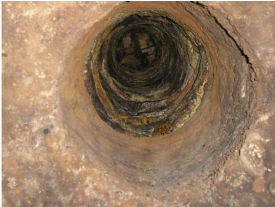
Ventilation shaft in a cellar in Mád
